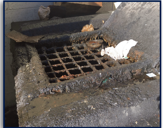
A poorly maintained grease recycling bin. The bin is open and has a thick build-up of used cooking oil and grease on the outside.
